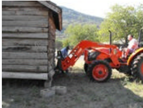
Workers leveled the CCC building as they placed it next to the Visitor's Center.
